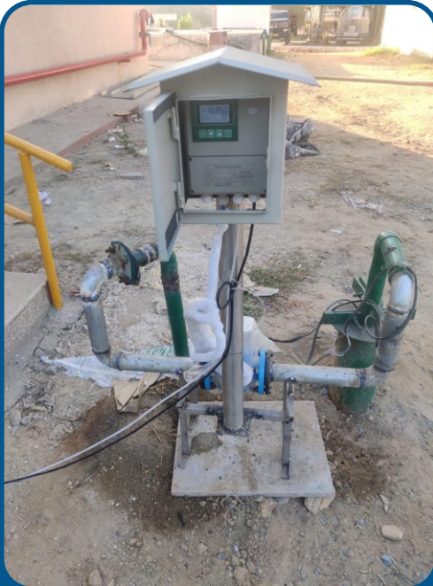
CGWA Monitoring System
